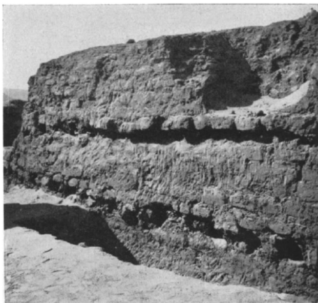
Fig. 1. The outer south wall of the storehouse-granary at Tell el-Kheleifeh, showing double row of apertures caused by burning and/or decay of horizontal wooden beams.
