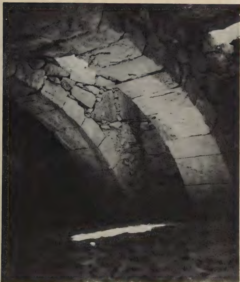
FIG. 40. Interior of a Nabataean-Byzantine covered cistern by the Wadi Siq in the Negev (see page 234).
