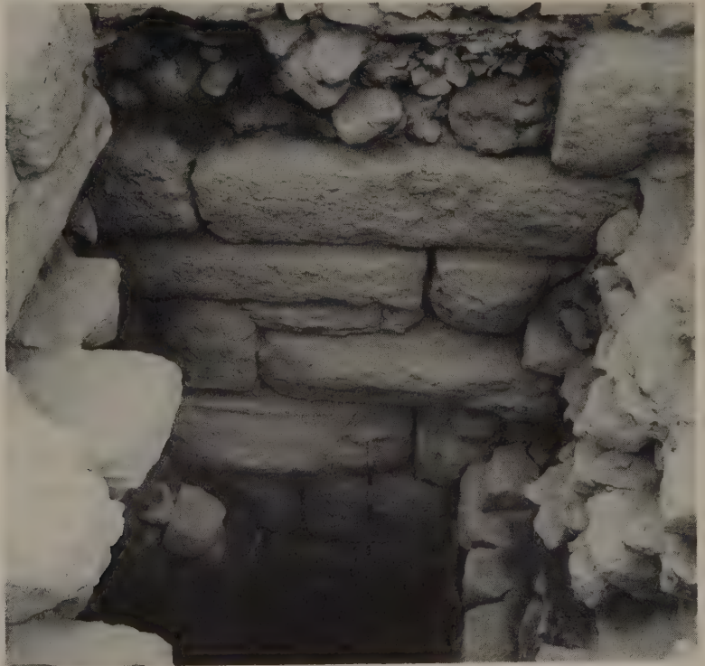
Pl. 27. Wall at Jerusalem, Site S II, containing re-used stones probably of Solomonic date.
