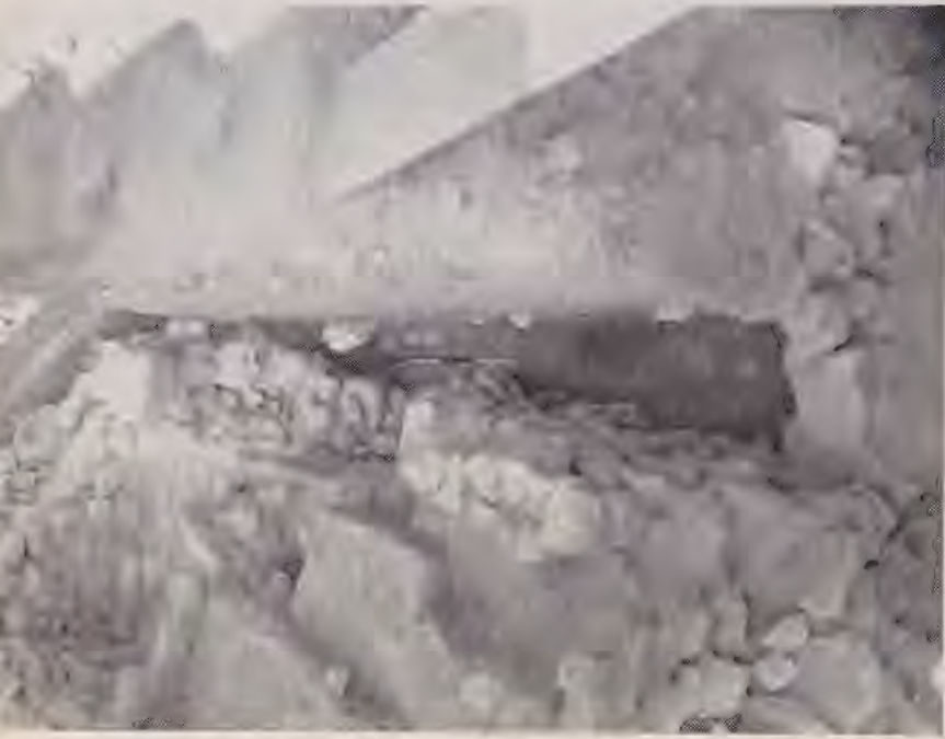
21 Interior terraces were supported by retaining walls parallel to slope of hill. This photograph shows how they bulged and collapsed (p. 95)
